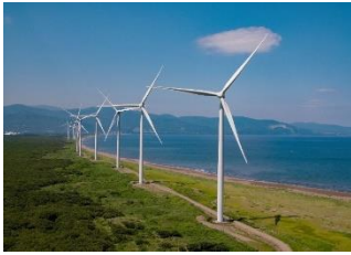
ReENE Zenibako Wind Power Plant (Otaru, Hokkaido)
