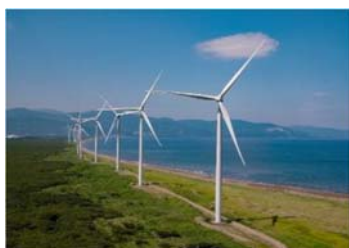
ReENE Zenibako Wind Power Station (Otaru City, Hokkaido)
