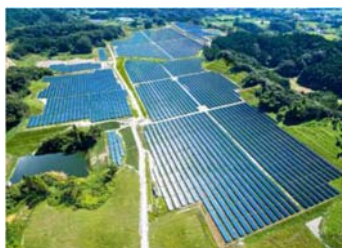
ReENE Naga Photovoltaic Power Station (Town of Chonan, Chiba)
