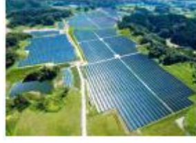
ReENE Chonan Solar Power Station (Chonan-cho, Chiba)
